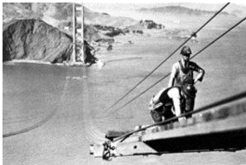
Workers on a catwalk during the construction of the Golden Gate Bridge. It would be completed in 1937.
